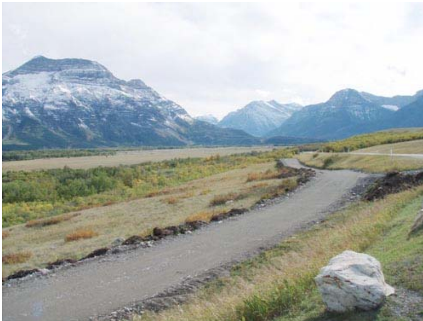
Construction of a walking and bike path along the entrance to Waterton Lakes National Park. Keith Hammer Photo.
