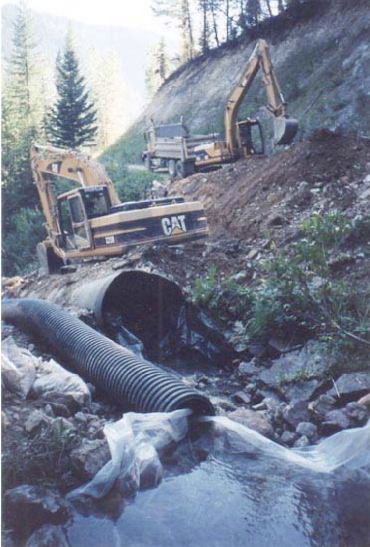
A culvert is carefully removed in the Quintonkin watershed of the Swan Range. Photo by Paul Harvey.
